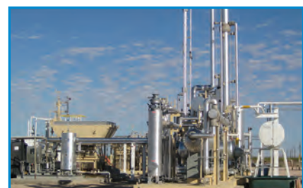
1.3 MMSCFD Natural Gas Processing Plant, Mentone, TX
