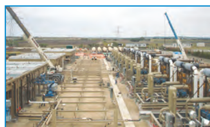
69,000 HP (9) Compressor Station
