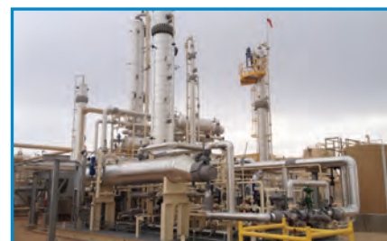
30 MMSCFD Natural Gas Processing Plant, Goldsmith, TX
